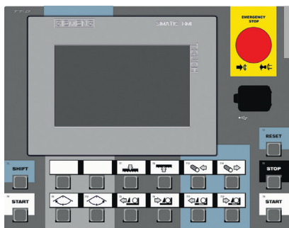
CONTROL PANEL: SIEMENS (X)
